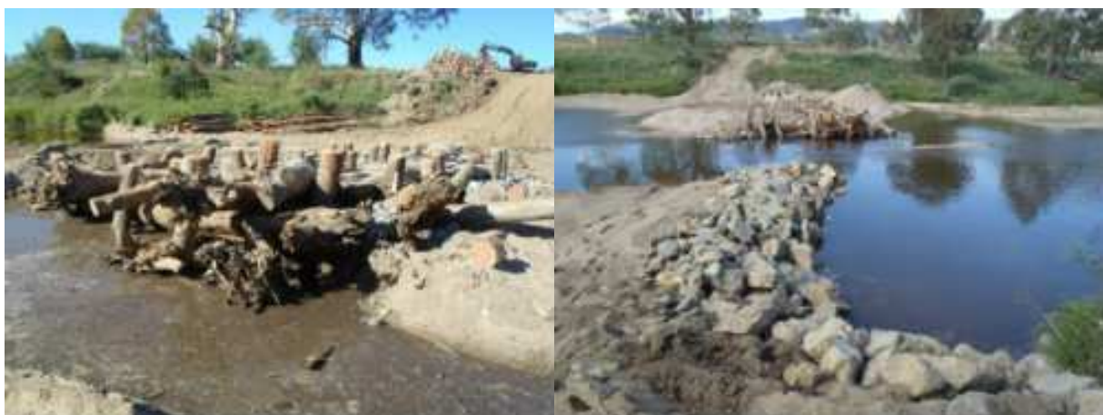
Figure 73. Left: ELJ placed prior to construction of rock groyne Right: Rock groyne constructed around ELJ (image courtesy of SCS, 2013).
